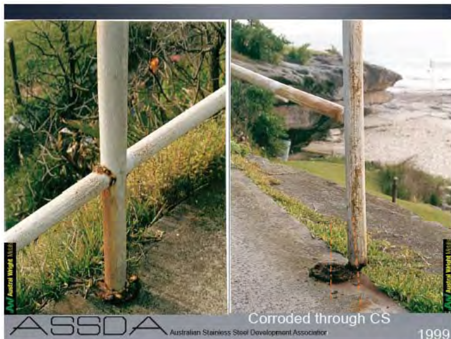
Figure 19.2 – Corroded Steel Handrail (ASSDA)
