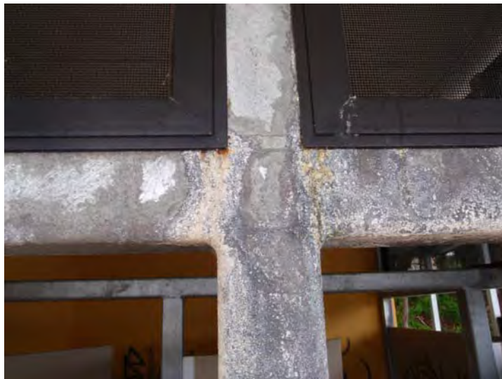
Figure 19.3 – Example of White Rust
